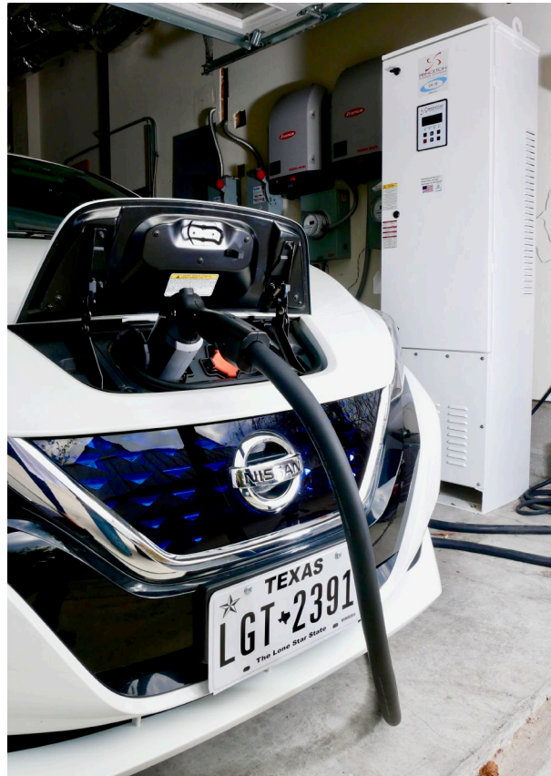
The V2G system at Pecan Street's Austin lab consisted of a Nissan Leaf with a 40kWh battery and a 10kW bi-directional charger. Pecan Street created custom code that allowed communication between the charger and the residential aggregator.
